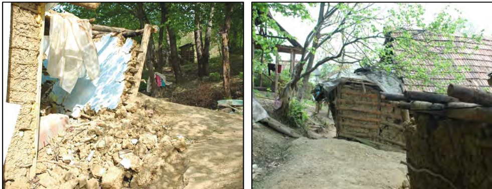
Fig. 4. Adobe houses damaged by the Chelintă landslide
